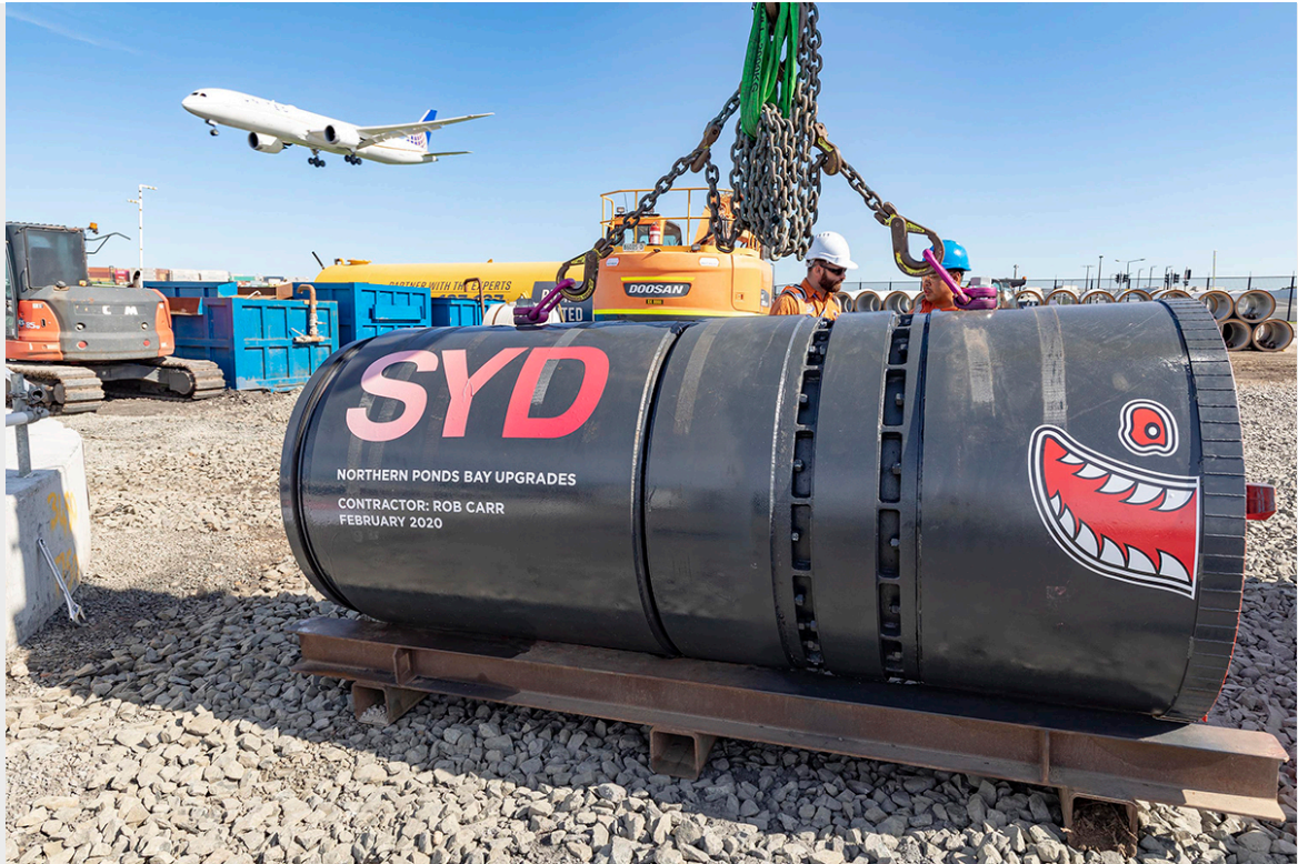
Northern Ponds Fuel Line, Sydney Airport
