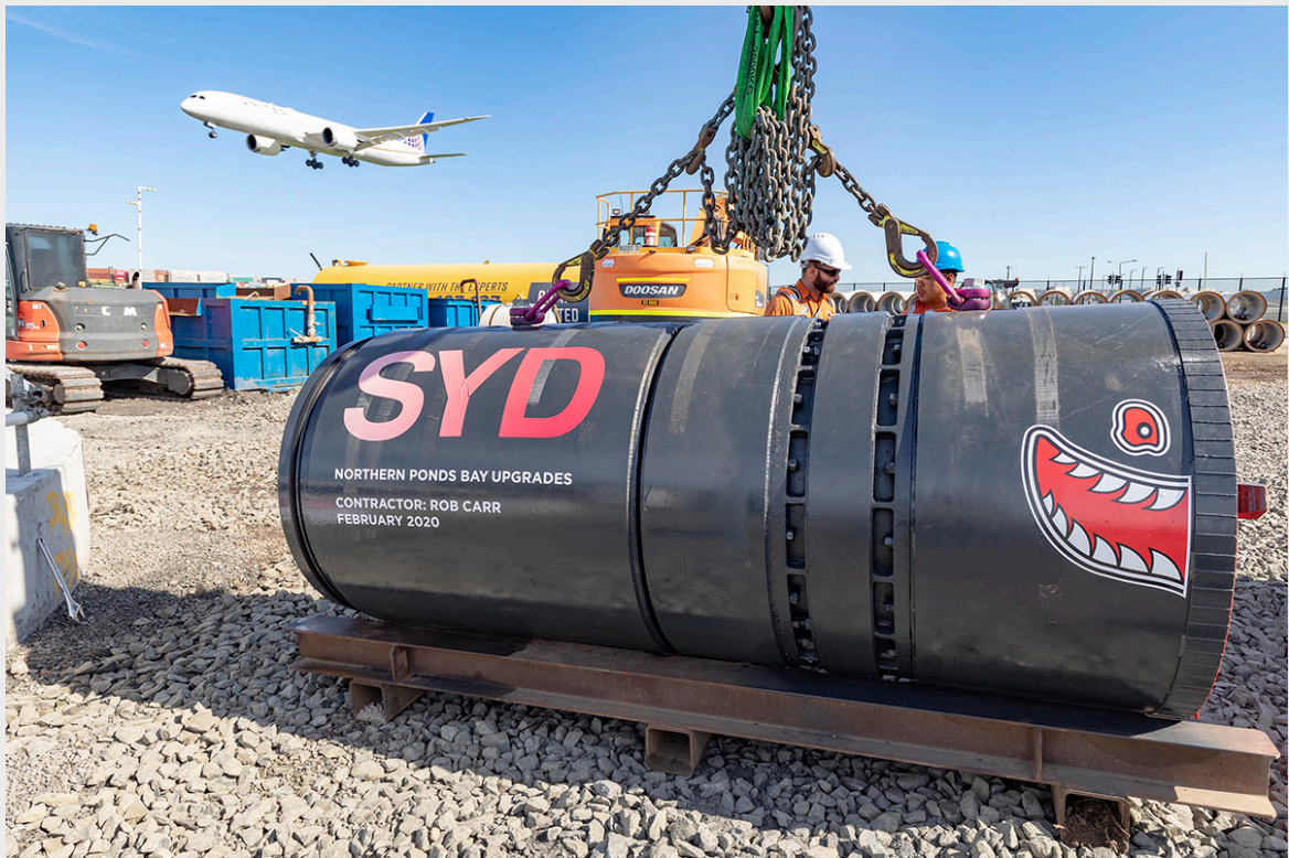
Northern Ponds Fuel Line, Sydney Airport
